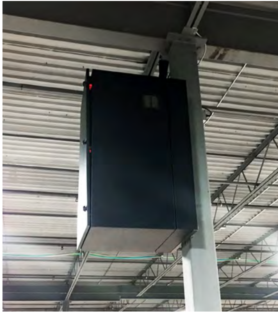
Figure 3: Standard Swing Wall-Mount Enclosure mounted overhead of a workspace. The fan was added to remove heat from network switches. This style of enclosure provides front and rear access to equipment.
