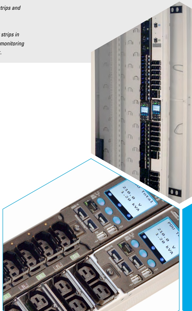
Figure 1: PDUs and Power Strips are used to distribute power into ICT racks and cabinets.
