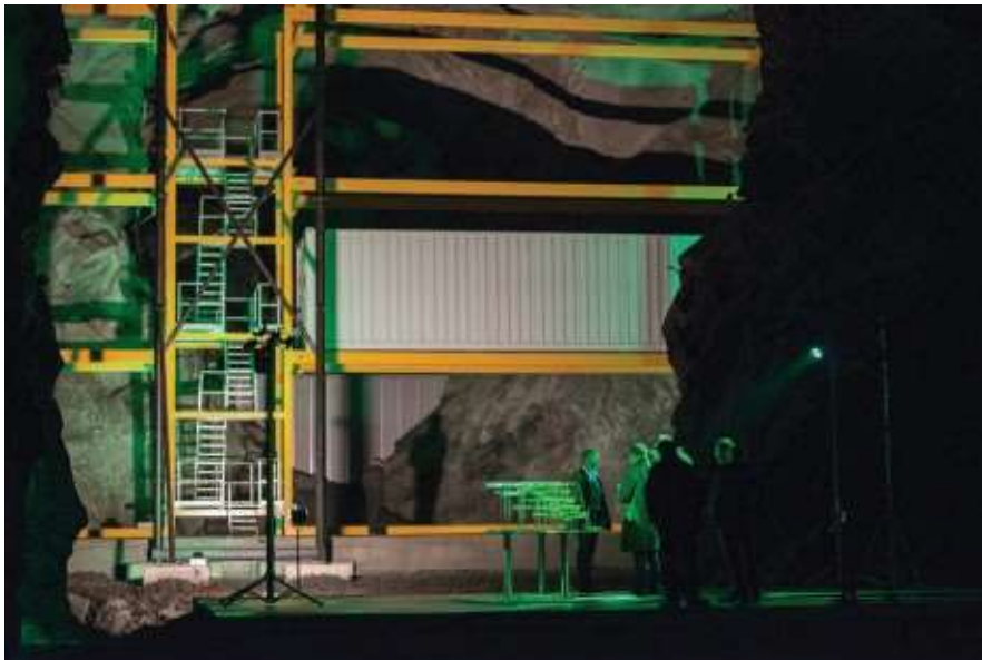
This photo was taken at the opening of Lefdal Mine Datacenter, May 10, 2017. The overall modular concept eventually will accommodate up to 1,500 containers with a cooling output of about 200 megawatts.
