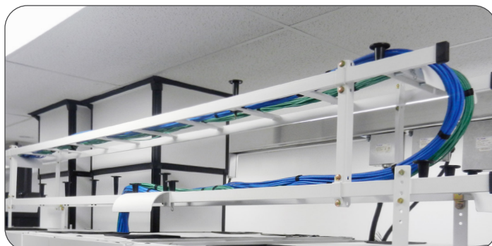
Cable Pathway Systems
