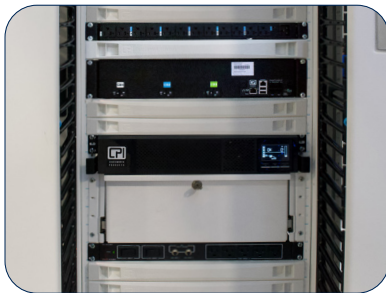
Rack power distribution units (PDUs) and uninterruptible power supplies (UPS) that can be monitored and controlled remotely
