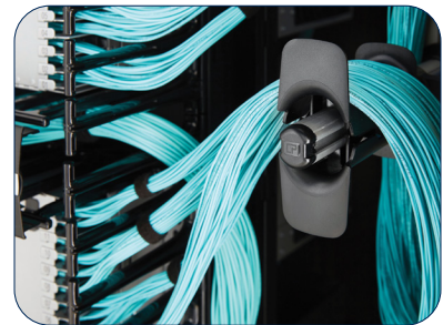
Cable management and pathway to organize high-density cabling
