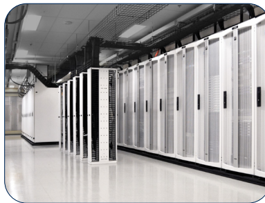
Server cabinets and racks to support and protect heavy equipment
