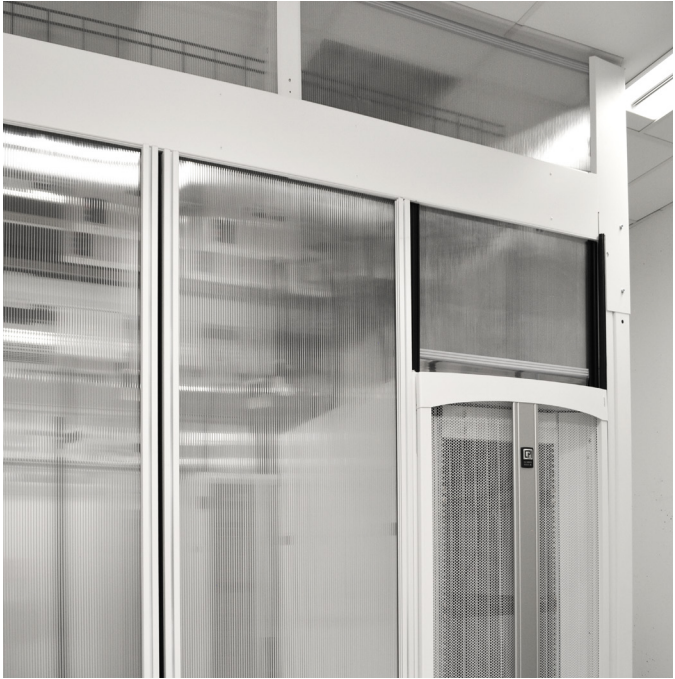
UF Health Shands utilized CPI’s custom HAC Solution to maintain cooling, while accommodating storage solutions of various heights, widths and depths.
