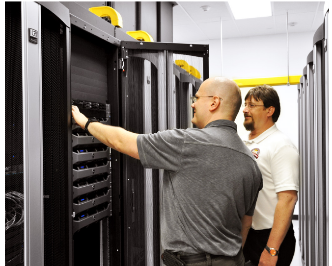
Robert Carneim, PhD, Supervisor of Instructional Technology and Doug Cofer, Data Center Director for Oak Ridge Schools chose CPI F-Series TeraFrame® Cabinets with Vertical Exhaust Ducts and custom grommets to keep the room temperature in their data center effectively cool.
