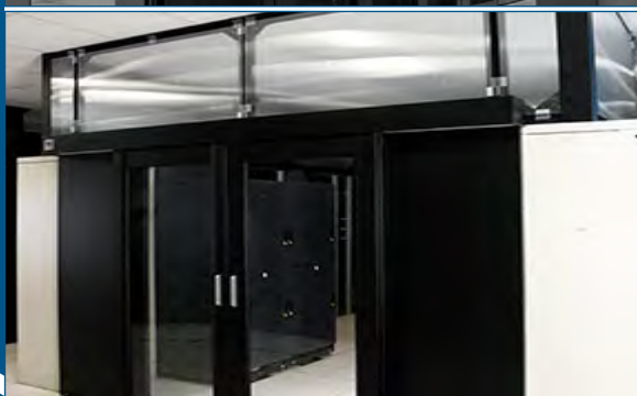
Figure 11: Hot Aisle Containment (HAC) typically uses a duct to surround the contained aisle. Hot air is isolated within and exhausted from the room through the duct.
