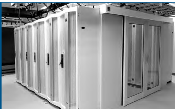
Figure 9: Aisle containment doors are available in various styles and widths. Ensure a good seal between the door frame and the sides of the adjoining cabinets. Consider a door that includes a mechanism to return and maintain it in a closed position.
